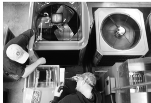
Daniel Knuckles (r) David Cox installing new R-41-A 16 SEER air conditioning unit
