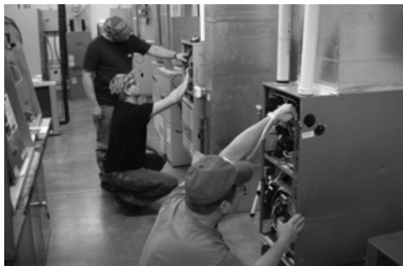
David Cox (front) Freddy Perry (middle) and Scotty Osborne checking gas furnaces
